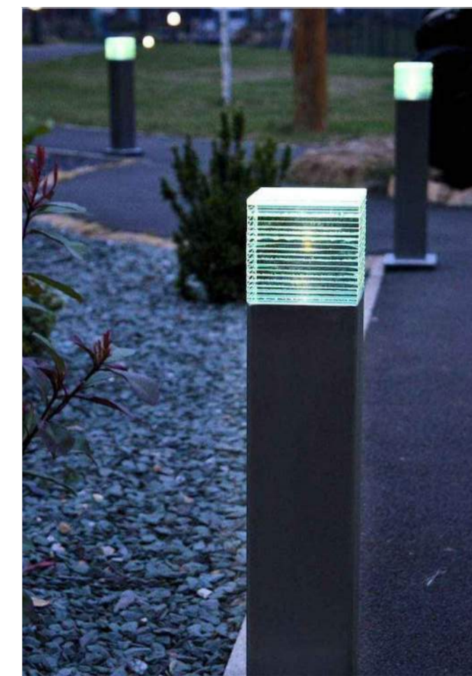
EDMONTON TRAIL AND 1ST AVENUE BOLLARD LIGHTS
